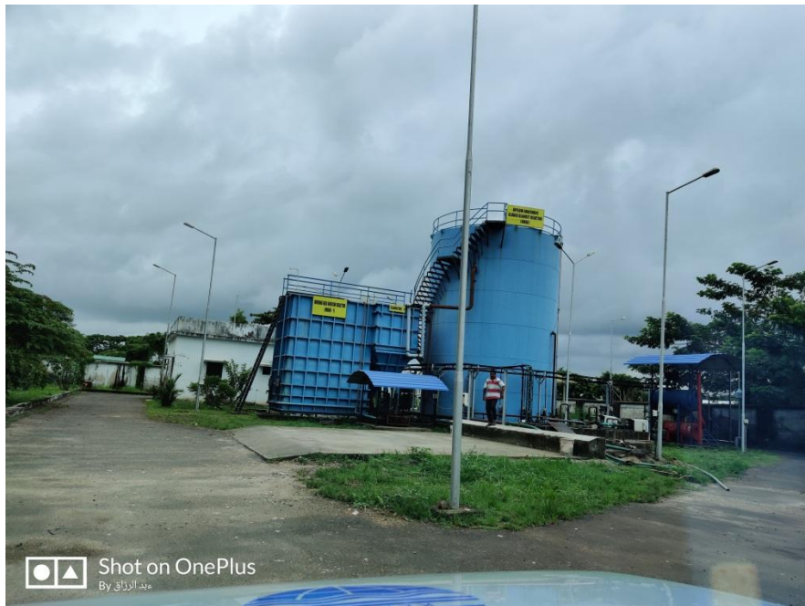
Fig.18.16 Septage treatment plant at Willingdon Island, Kochi, Kerala
