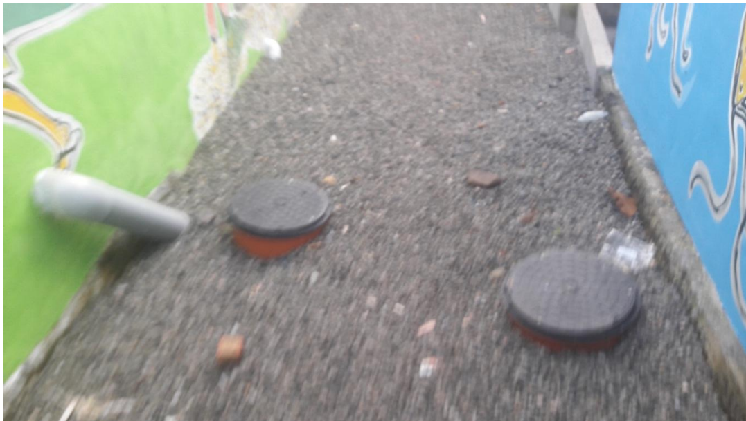
Fig.18.21 Manholes in the pipe lines
