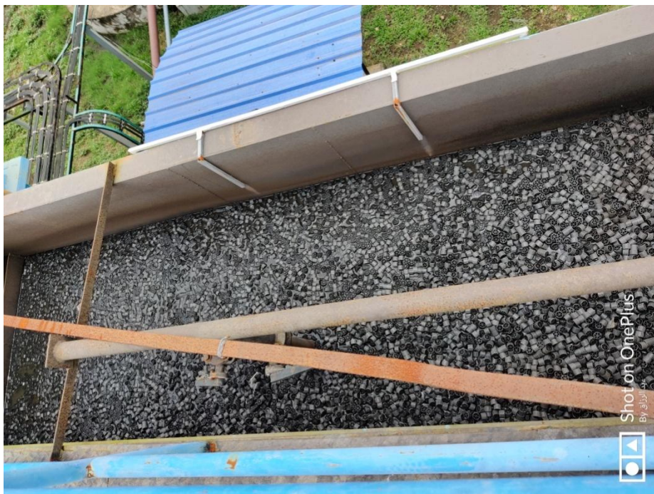
Fig. 18.17 Moving Bed Bio Reactor in the Septage treatment plant, Willingdon Island
