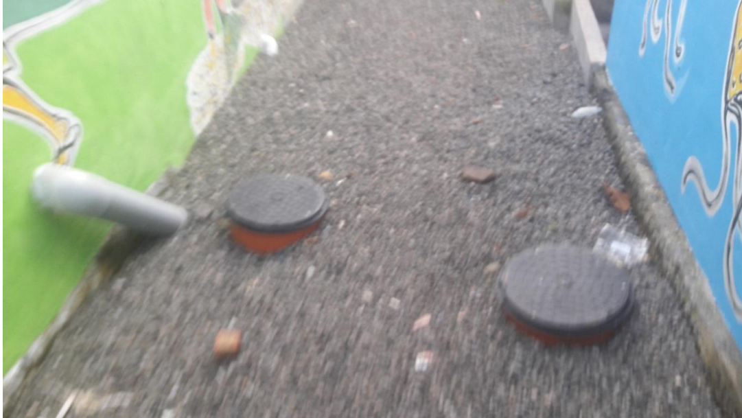
Fig.18.21 Manholes in the pipe lines
