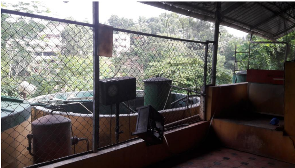
Fig. 18.12 Biogas plant in TechnoPark
